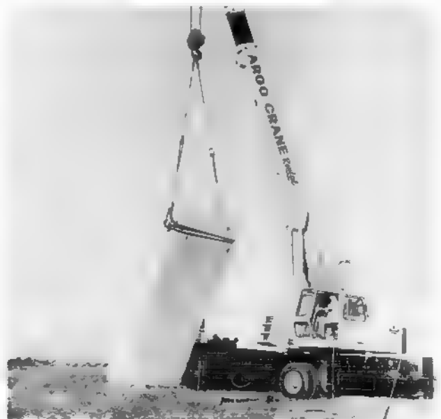
A Guidestone granite slab is shown being hoisted from the transporting truck by Grady Albertson, owner and operator of Argo Crane Service. This is the first of The Georgia Guidestones® to arrive at the erection site and its placement atop the foundation will mark history for it is the first known 'Message to Mankind' ever to be erected in the United States of America. Its purpose, as told by the sponsors is to leave a message, etched in granite that will survive the ravages of time.
